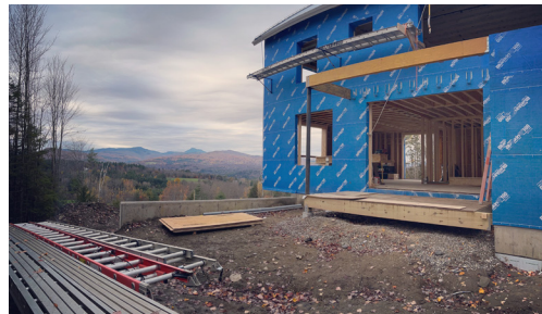
VGBN hosted a Green Building Construction tour of high performance homes and innovative affordable housing development in the Mad River Valley in October 2023.
